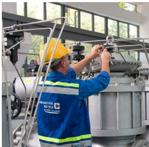
Image courtesy of GDF SUEZ Energy Romania.
